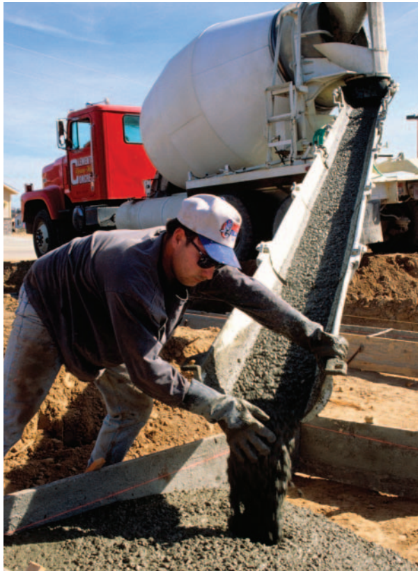
Figure 8-2 A Concrete Foundation Placing Concrete Concrete is delivered to the job site and placed into foundation forms.
