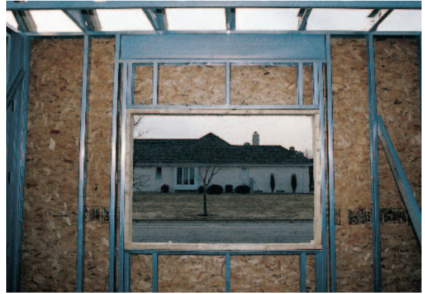
Figure 29-42 Rough Openings Rough Opening for a Window Note position of header in wall.
