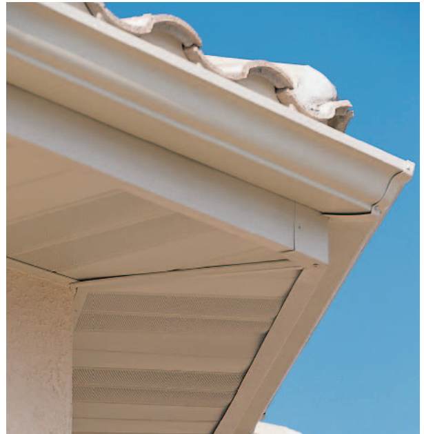
Figure 29-56 Enclosed Soffit Horizontal Method An enclosed soffit with ventilation openings. What is the purpose of the ventilation openings?
