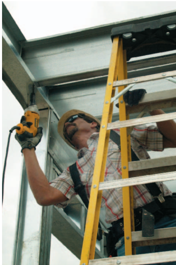
Figure 29-31 Floor Joists and Joist Tracks On Track Fastening the floor joists in the joist tracks.
