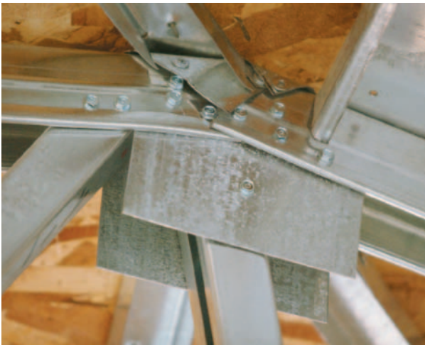
Figure 29-50 Heel Gusset Site Built Using a heel gusset to join the chords.
