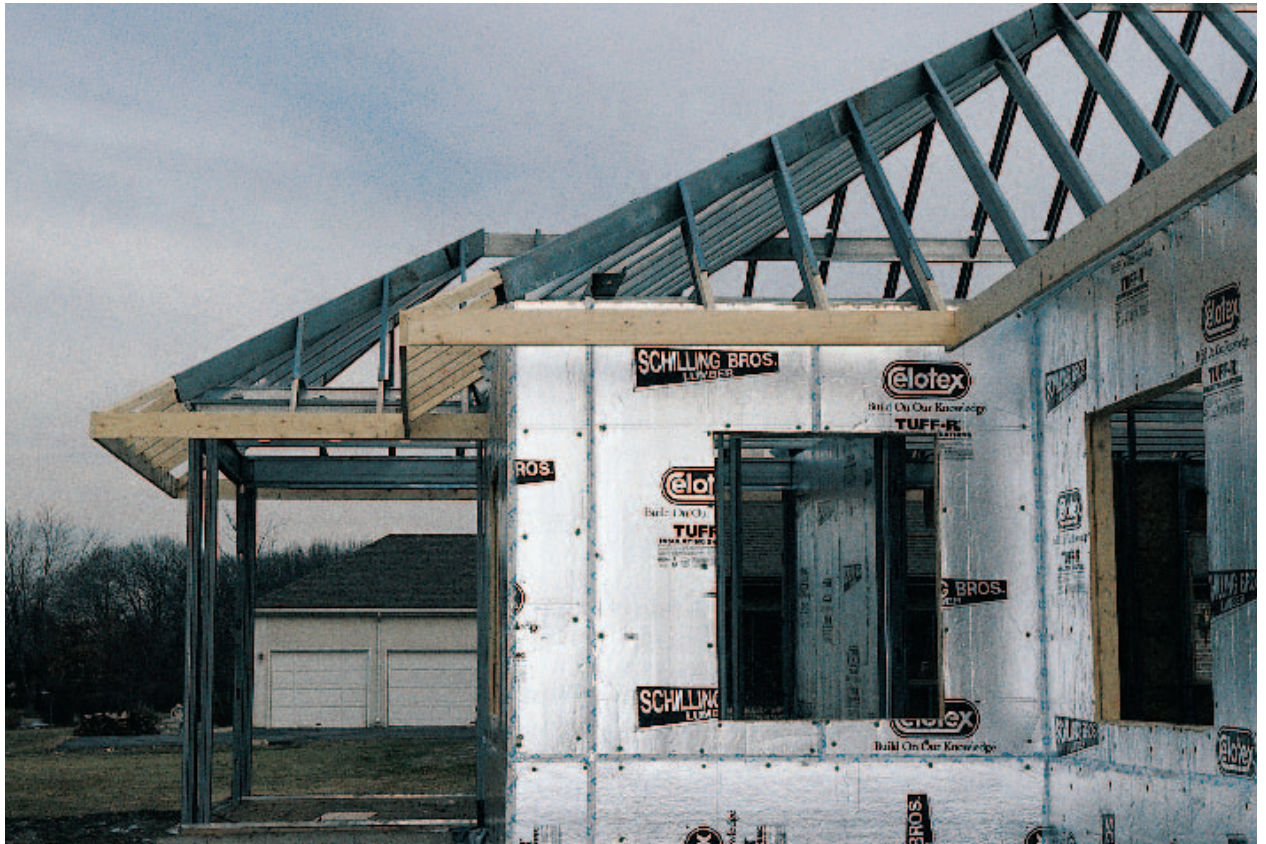
Figure 29-52 Fascia Plumb Fascia framing that is parallel to the side of the house.
