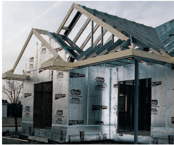
Figure 29-54 Roof Rake Extended Rake A roof rake extends beyond the house walls.
