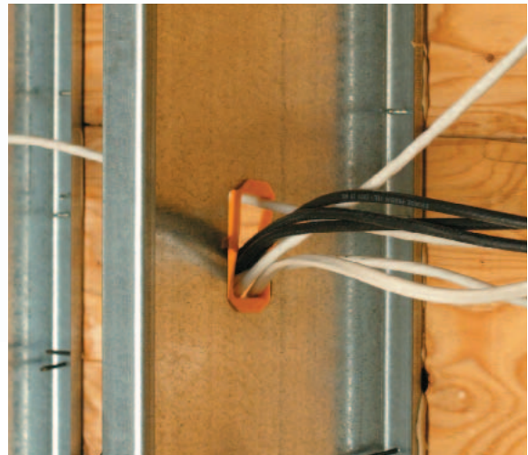
Figure 29-43 Punchouts Aligned Punchouts are aligned for straight runs of electrical wiring. Notice the grommets that cover rough edges.
