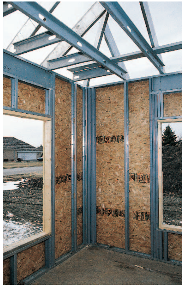
Figure 29-37 Bracing an Exterior Wall Panel Bracing Sheathing can brace an exterior wall and prevent twisting and racking.
