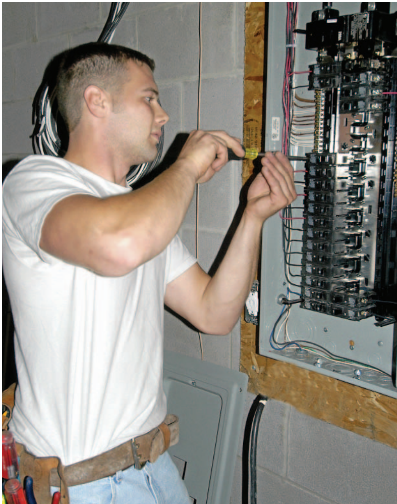
Figure 30-14 Service Panel Distribution Center Circuit breakers are located in the main service panel. Never work on the panel unless you are absolutely certain that power is not being supplied to it.
