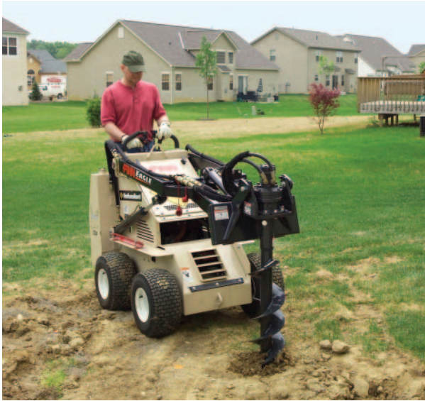
Figure 35-9 Excavation Quick and Precise The use of heavy equipment to drill holes for piers improves their accuracy and speeds the work when many holes are required.
